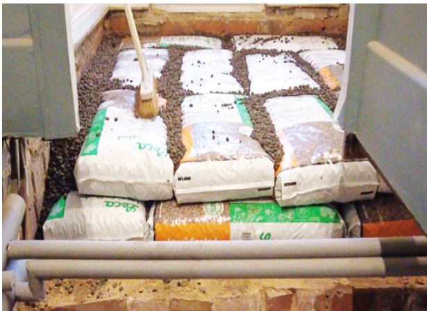
Step 3 30 Minutes Use loose material to fill any voids & level the surface
