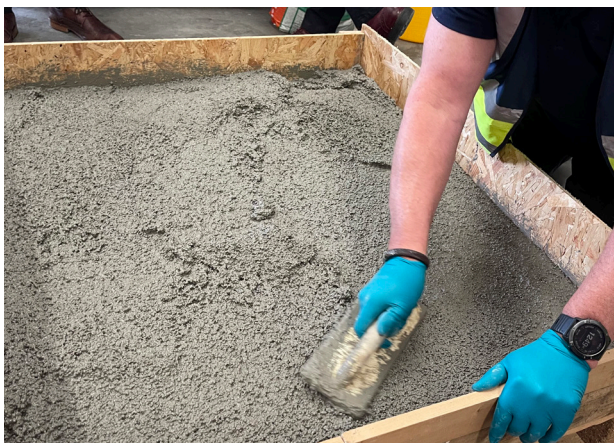
Step 5 60 Minutes Level to the desired thickness (4cm minimum) using a level and regularize with a manual or electric trowel
