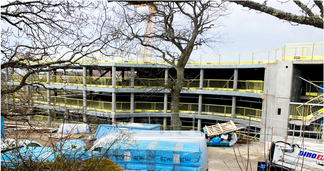
The parking structure was adapted to preserve the oak tree and protect local biodiversity.
