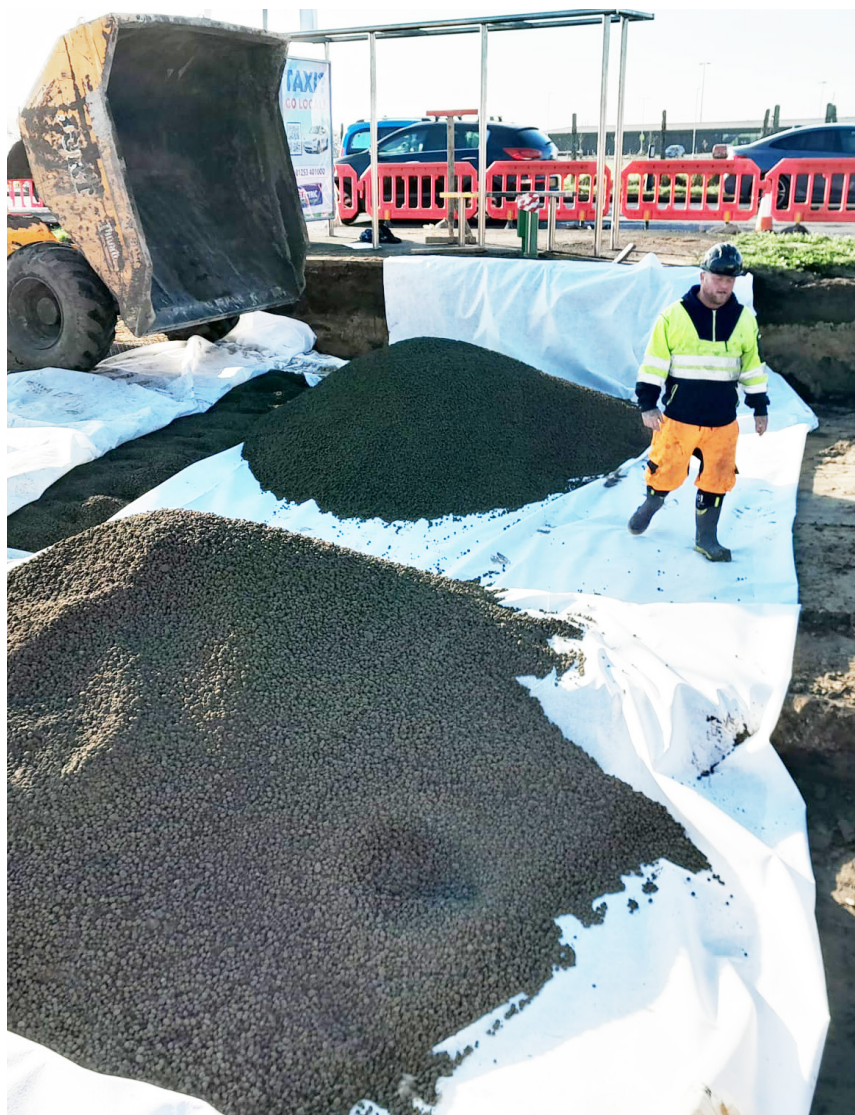
Leca LWA was chosen as a lightweight fill material, significantly reducing load-induced settlement.
