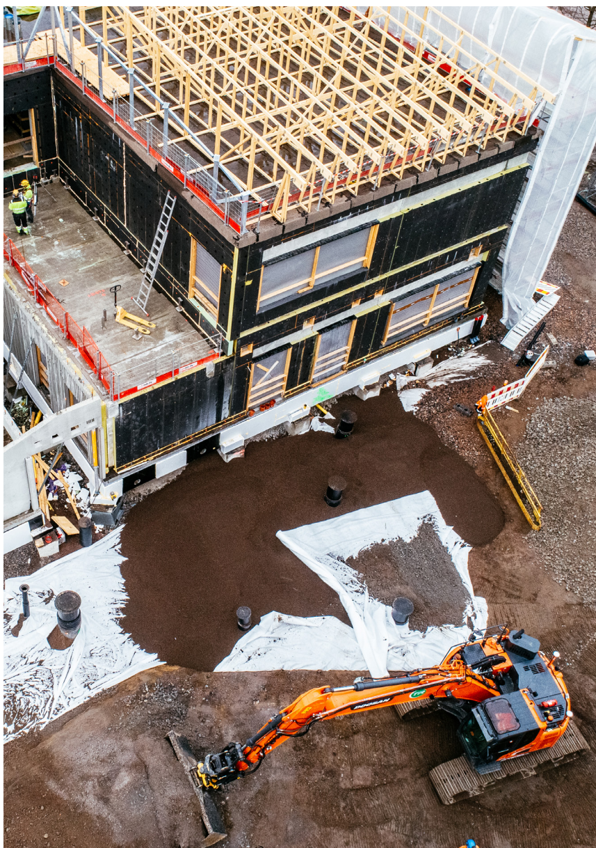
Over 2,000 m 3 of Leca LWA was used for the lightweight fills at Puotila School.
