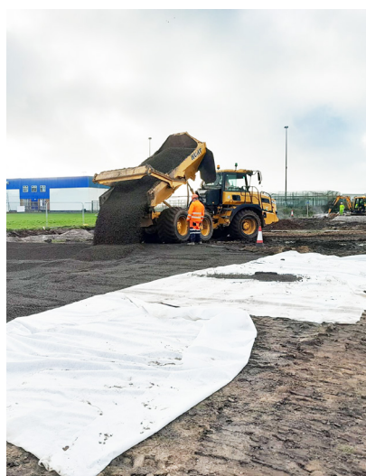
The presence of soft ground made conventional construction methods unsuitable for the project.
