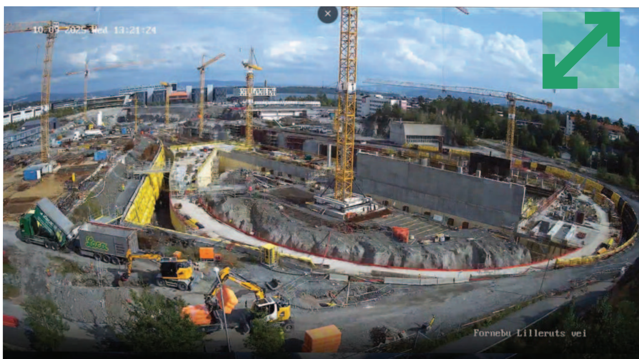
Leca® LWA is blown into place to reduce earth pressure around the new Fornebu metro station in Oslo.
