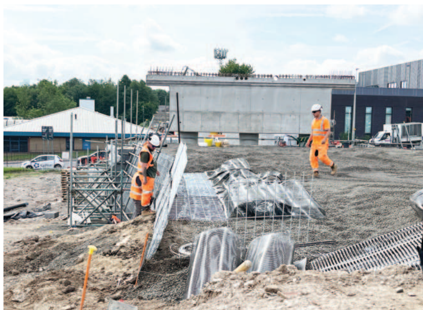
Lightweight fill required to reduce settlement risk and structural load on bridge abutments.
