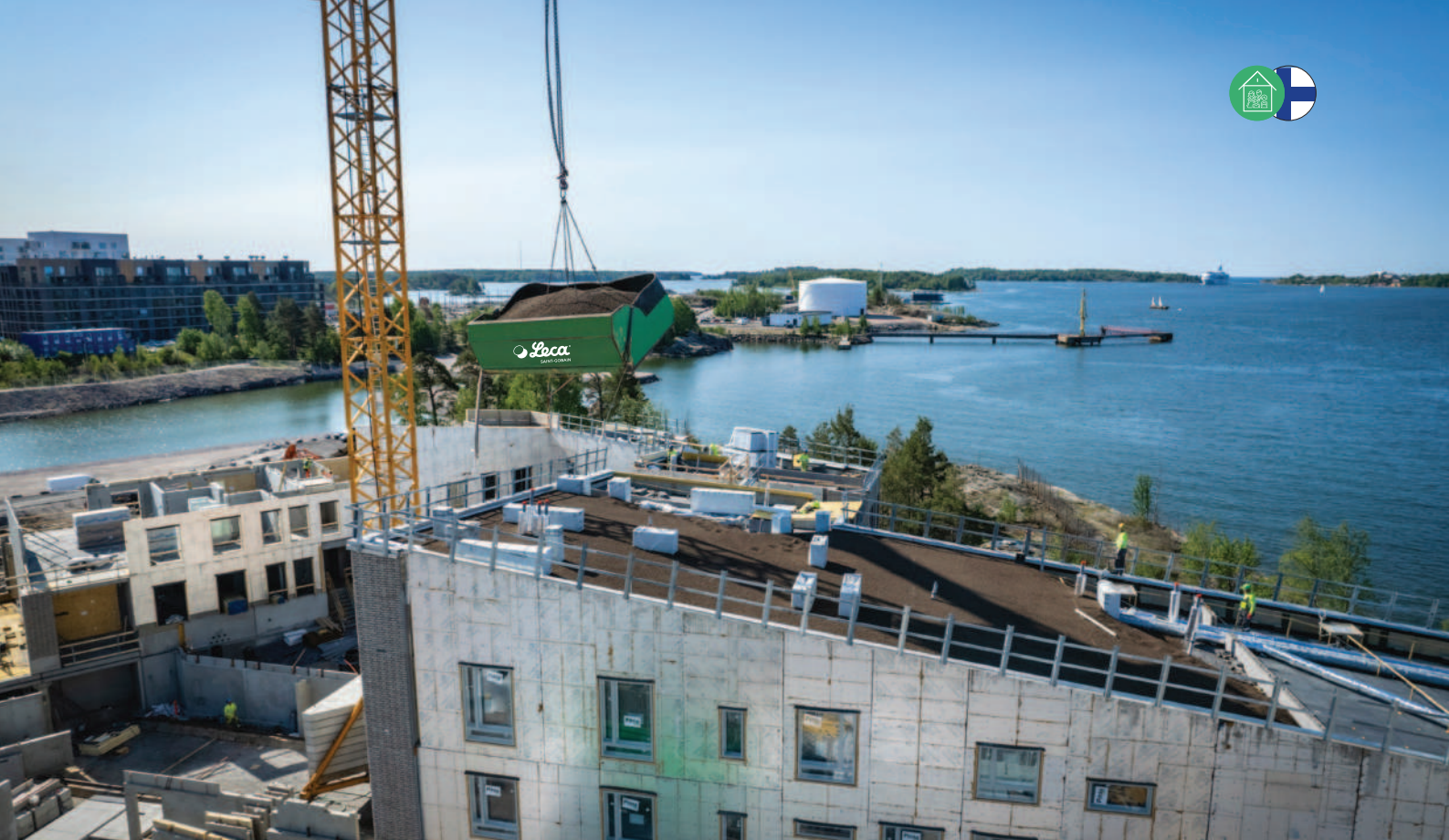
Lightweight aggregate was delivered to the roof (5–9 storeys) using a lifting box, supporting efficient installation on site.
