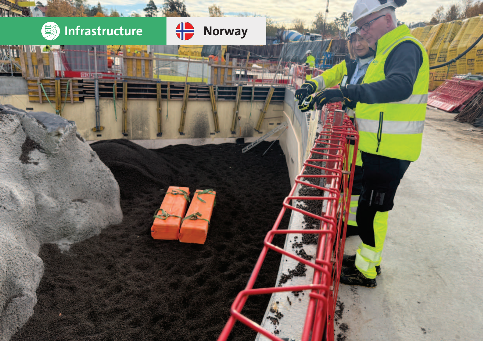
Representatives from Leca visiting the project site to inspect the installation of Leca® LWA, used to reduce earth pressure and improve safety and efficiency in a confined construction area.
