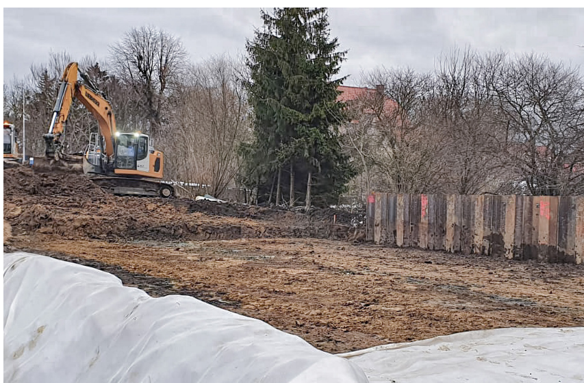
A protection of the track bed crown was constructed in the form of a retaining structure made of a sectionally anchored steel sheet pile wall.
