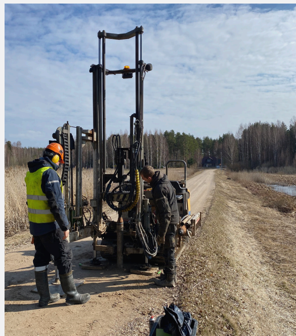
Test drilling in March 2024 to assess the condition of Leca LWA in the Varska road embankment.
