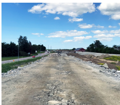
Earthworks for the new highway, improving capacity and safety for the 15,000 vehicles passing daily.
