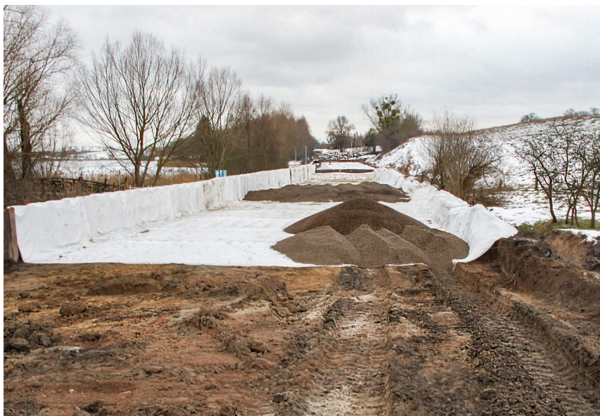
It was decided to use a geomattress made of Leca® GEOTECHNICAL EXPANDED CLAY 8/10-20RX.”
