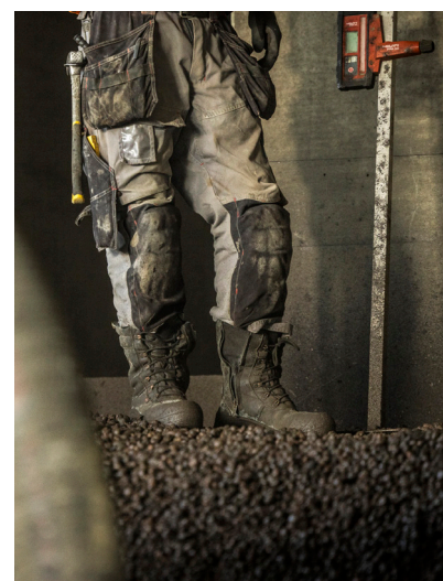
Leca blown into place, straight from the truck, fully compressed - no need for manual unloading, no problems to walk on and zero packaging.
