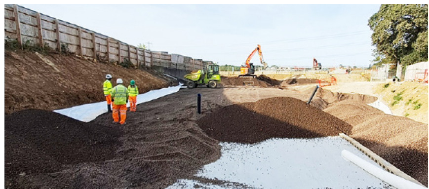
Over 5,600m 3 of Leca LWA supported the culvert extension before earthworks began.
